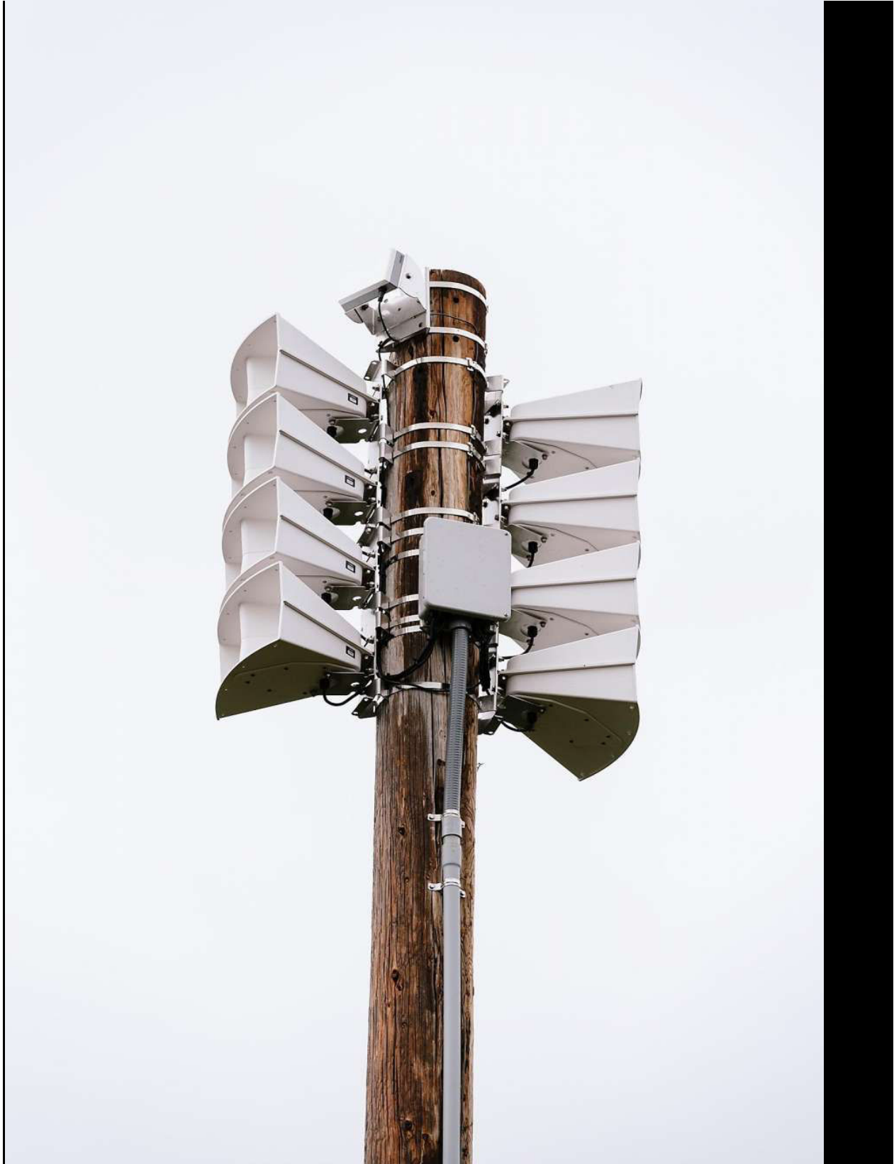
One of Mill Valley's five new LRAD satellite-based siren notification emergency systems in Mill Valley, California, Saturday, December 7th, 2019. Photo: Michael Short
